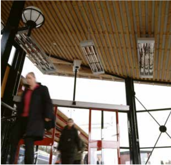
This train station outside Stockholm is heated by IR. A control with timer allow waiting passengers to increase the heat when it is particularly cold.
