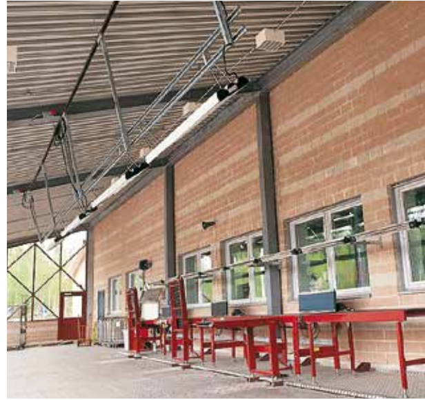
The IR heater can be mounted in an angled position to direct the heating where it is needed. Heaters used outdoors should be placed under a roof. In this installation the working stations are heated by IR heaters in the ceiling and CIR heaters on the wall.
